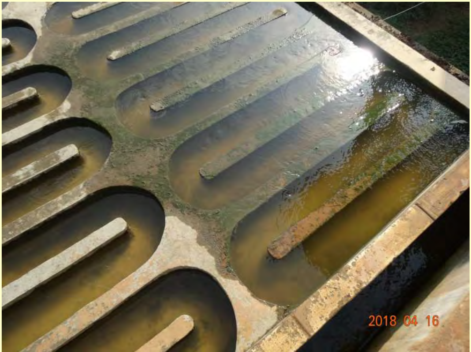
Baffling type flocculation basin with no flow, overflow, and algae attachment
