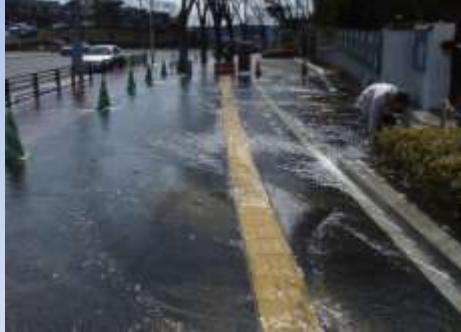
SP \phi 600 leakage
