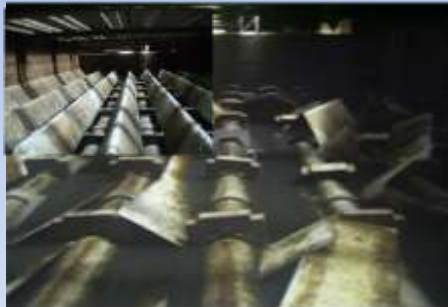
Damage to the sedimentation baffle boards.
