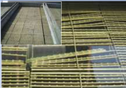
Damage to the sedimentation inclined basin plates.
