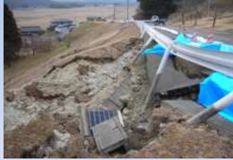
Slope failure in Fukuoka Water Purification Plant
