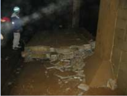
Collapse of flow arrangement wall in Anyoji Distribution Reservoir
