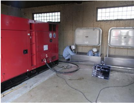
Generator was installed, and then started to supply water at Takegoma water resource in Rikuzentakata City (May 10)
