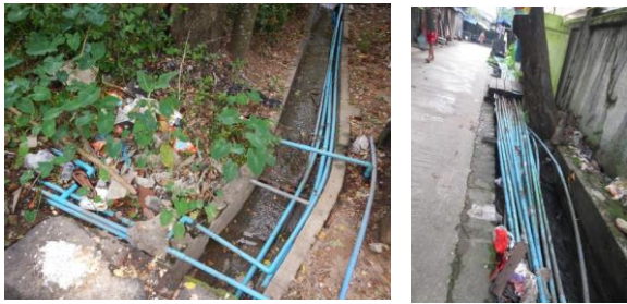
Figure 2 Several service pipes in parallel on the ground
