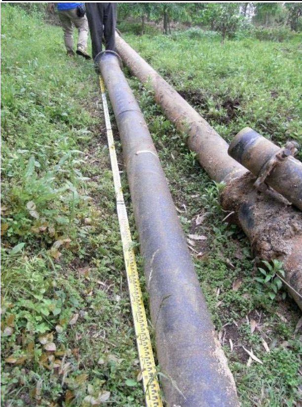
Damaged DIP of D200, and D150 (K type) (Mashiki Town, Fukuda District) Distortion of the pipe shows how large stress put on the pipe
