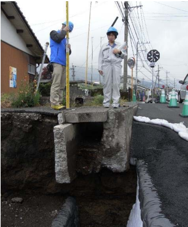
(Upper and lower) Surface faulting appeared in Kario District, Aso City. Faulting was 40~50 m wide, 1.6~2.1 m of displacement height, and 1 km long in total.
