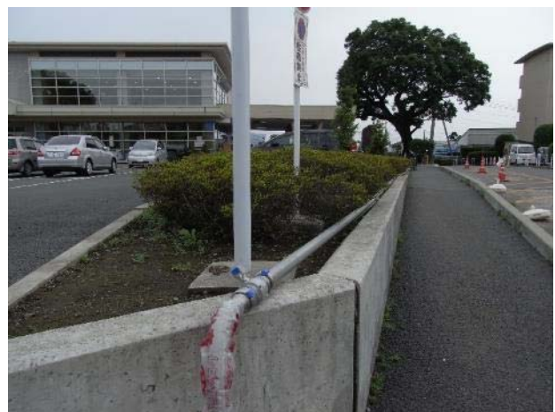
Temporal water service pipe supplying to the Mashiki Health and Welfare Center, temporarily used for an evacuation shelter.
