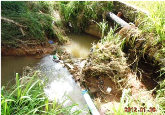
Photo 3: Underground water flowing into pipe
