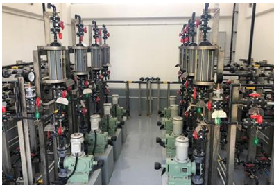
Dosing facilities of sodium hypochlorite, Nyaunghnapin WTP
