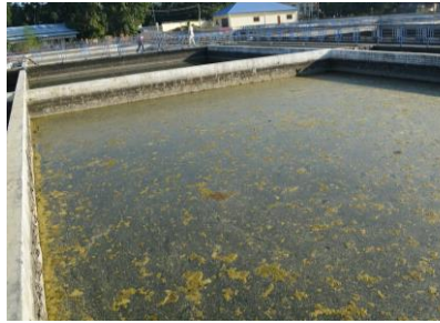
No.8 WTP of MCDC, algae in receiving tank
