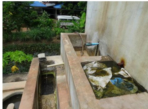
Fig. 3 Water purification plant full of garbage
