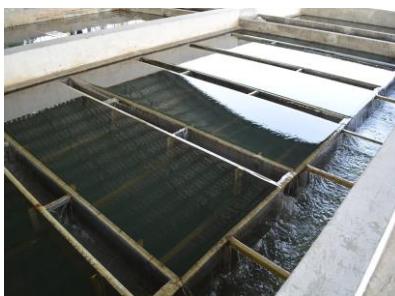
Well-functioning settled water collecting basins, No.4 WTP in Mandalay
